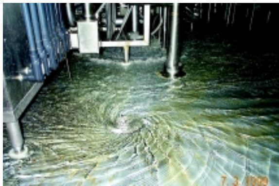
An example of one source of needless waste of water, chemicals and energy in a food processing plant. The overflow resulted from an inefficient Programmable Logic Control (PLC) system controlling a Reverse Osmosis Cleaning-In-Place process.
