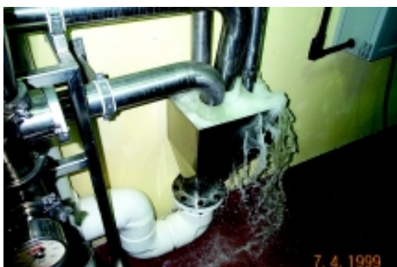
An example of water being wasted at an evaporator system due to defective controls, causing clean water to be diverted to the drain instead of the water recycling system.
